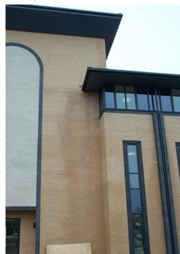
Design detailing has caused saturation staining where water runs off roof ledges.
