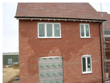
Saturation occurring prior to roof & window placement.
